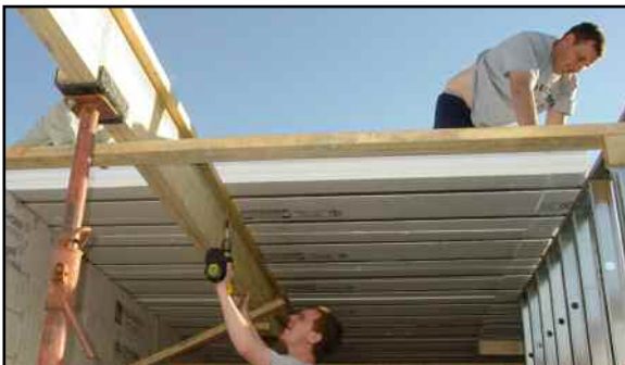
Shoring must be attached to the wood rib of the LiteDeck sections.
