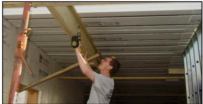
Shoring must be attached to the steel rib of the LiteDeck sections.
