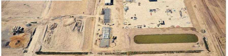
The largest project that Dickinson has poured to date is the Baker-Hughes Frac Station in 2011, which required 25,000 yd. of concrete and included seven buildings and nearly 900,000 sq. ft. of 8-in. concrete paving. This aerial shot shows the facility under construction and Dickinson's portable RexCon plant (lower-left corner) and arrival in North Dakota (inset).
