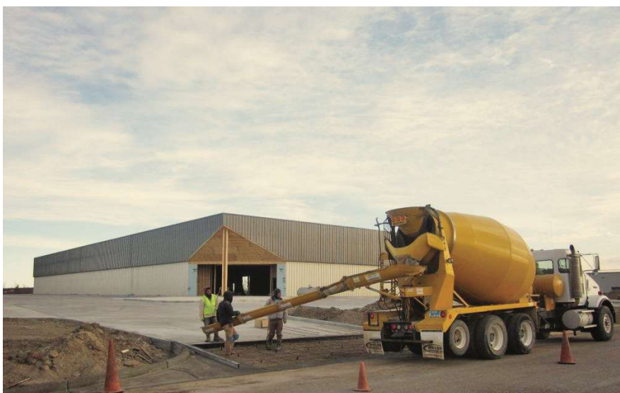
In partnership with various contractors, the company has successfully promoted the pouring of many concrete parking lots in the area. Dickinson provided material to Winn Construction for this 62,000-sq.-ft. parking lot at a commercial project in the town.
